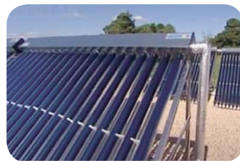
6. Solar panels producing heat
